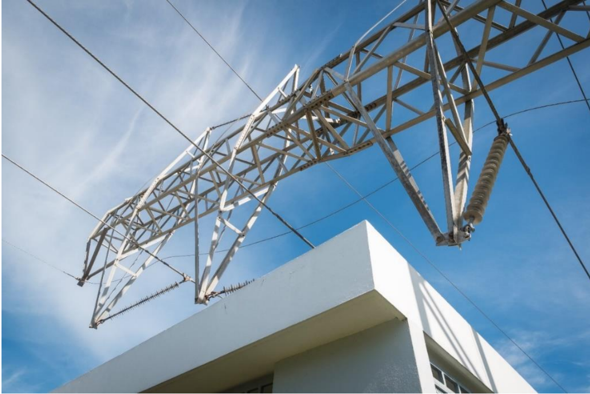
Figure 24 - Guaynabo, Puerto Rico – Power lines remain broken and down along roads and residential areas nearly three months after Hurricane María
